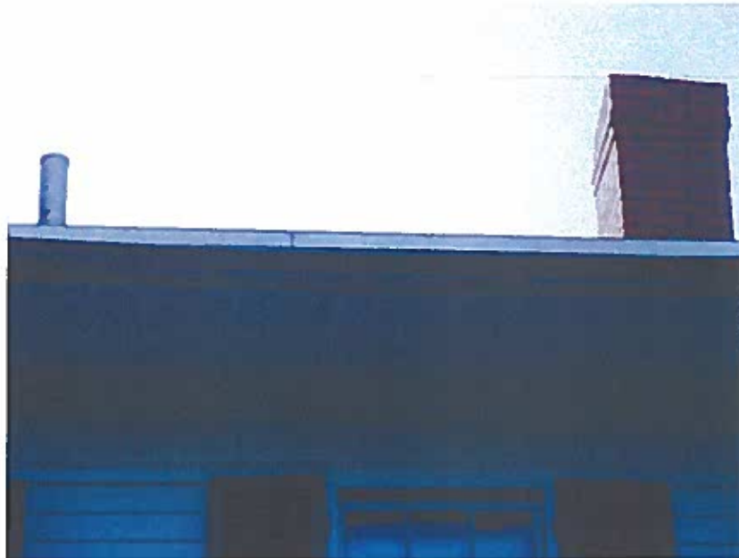
Photo 2: Close up view of roof. Note loose gutter.
