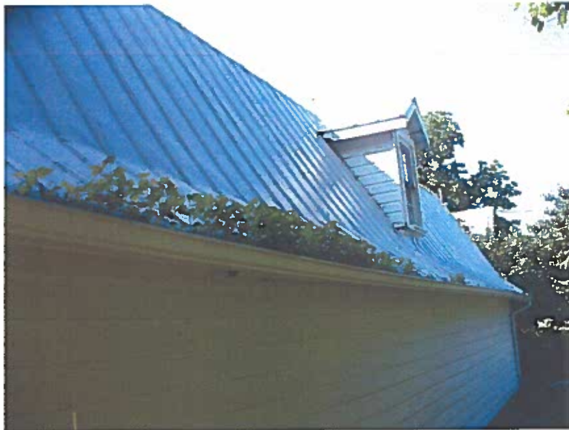
Photo 2: Close up view of roof. Note plant growth in gutter.
