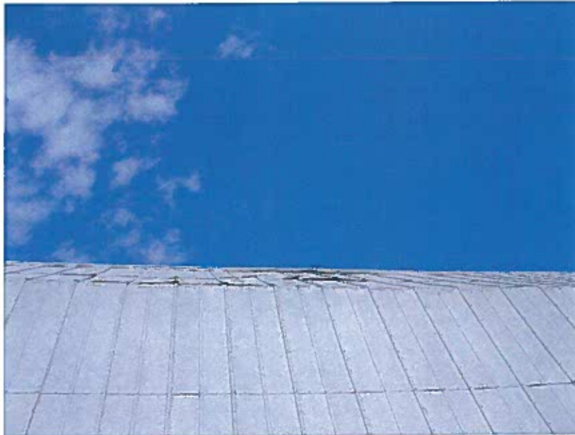
Photo 2: View of roof. Note loose roof panels.
