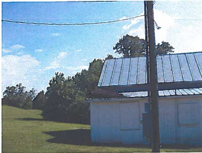
Photo 2: Close up view of roof. Note poor condition of BUR.
