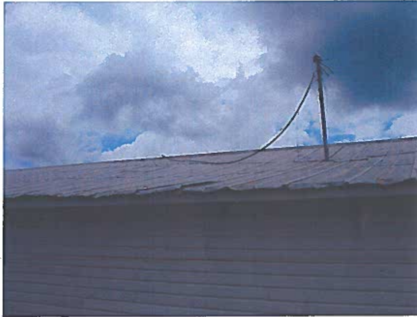
Photo 1: View of roof. Note loose roof panels and belly in roof.
