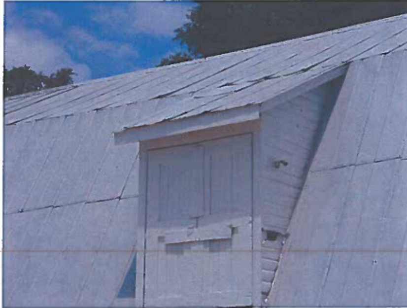
Photo 1: View of roof. Note unattached roof panels
