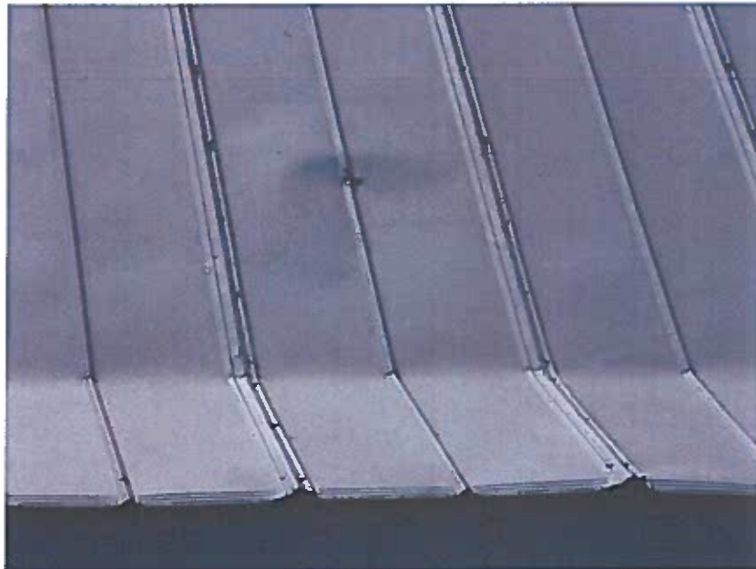
Photo 2: View of hole in roof.
