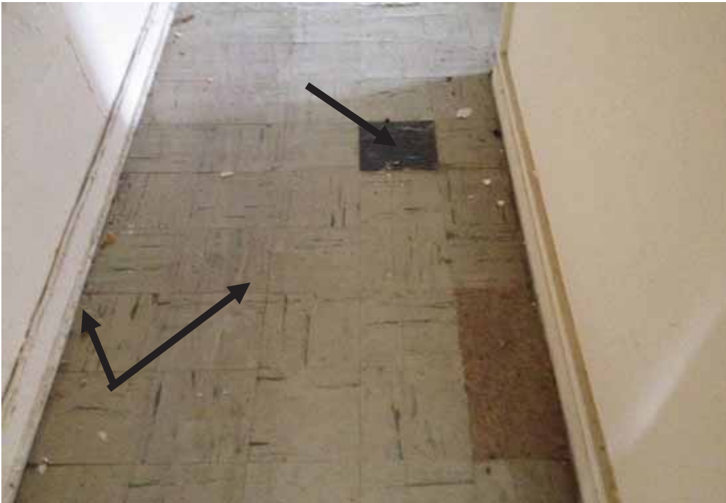
Photograph No. 4 Asbestos containing floor tiles in the garage (2)
