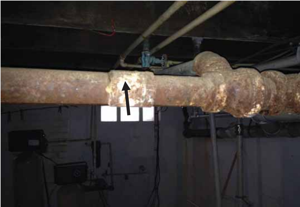
Photograph No. 8 Residual pipe mud on elbows and joints in the basement (1)
