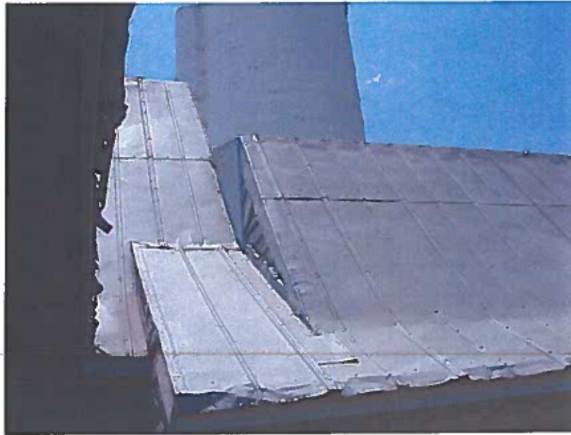
Photo 1: View of roof. Note bent roof panels
