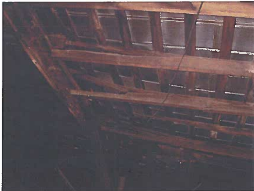
Photo 2: Interior of building. Note broken structural supports
