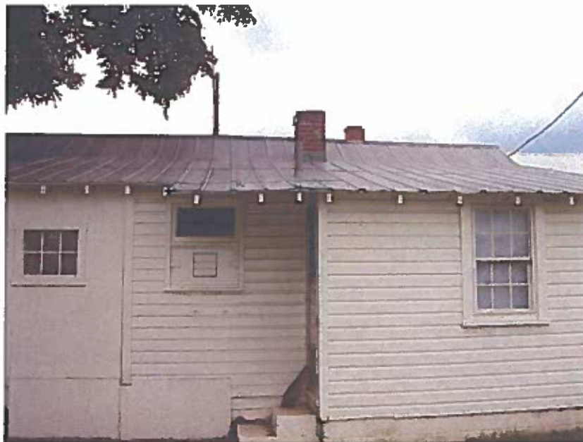
Photo 2: Close up view of roof. Note covered chimney and general condition of roof coating.
