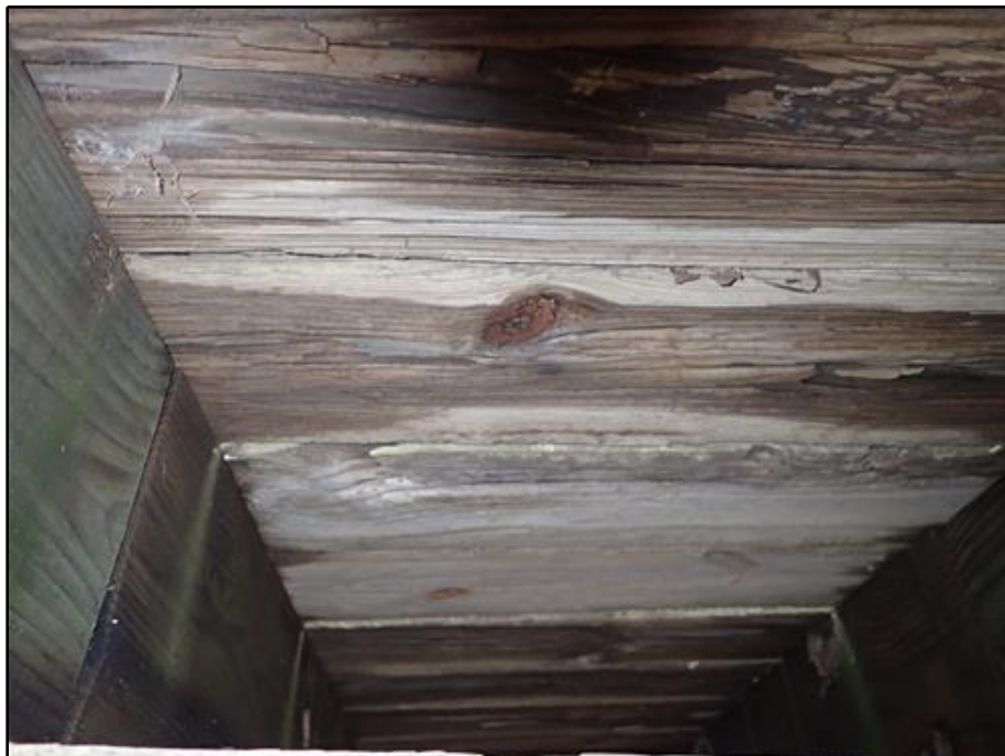
32. Underside Span 3 - Four Planks with Rot/Decay in a 3 ft. Width (Plank 1 is Worst)
