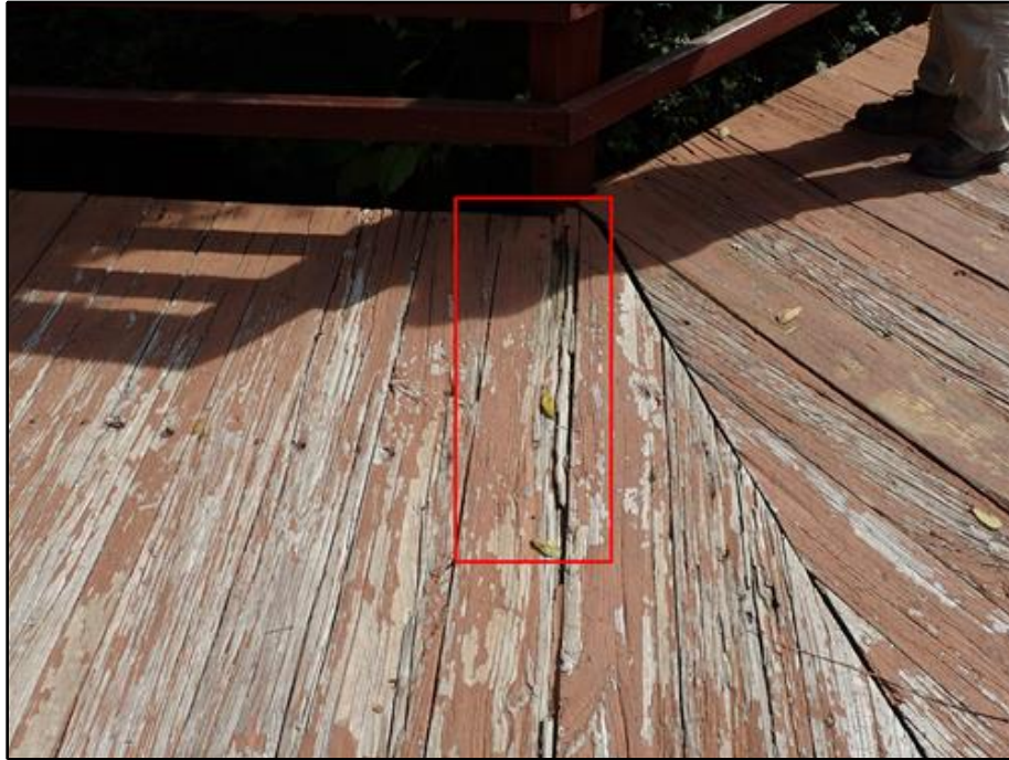
13. Span 3, Plank 14 - Full Length of Decay with 3/4 in. Pick Penetrations; Plank is also Loose
