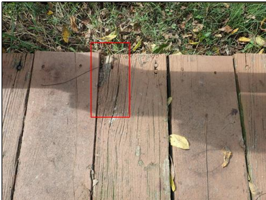
20. Span 14, Plank 13, South End - 3 in. Edge Splintering
