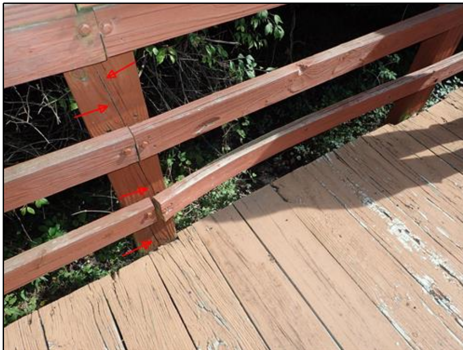
24. Span 5 - Warped Lower Rail Member of North Railing; Vertical Check in Rail Post
