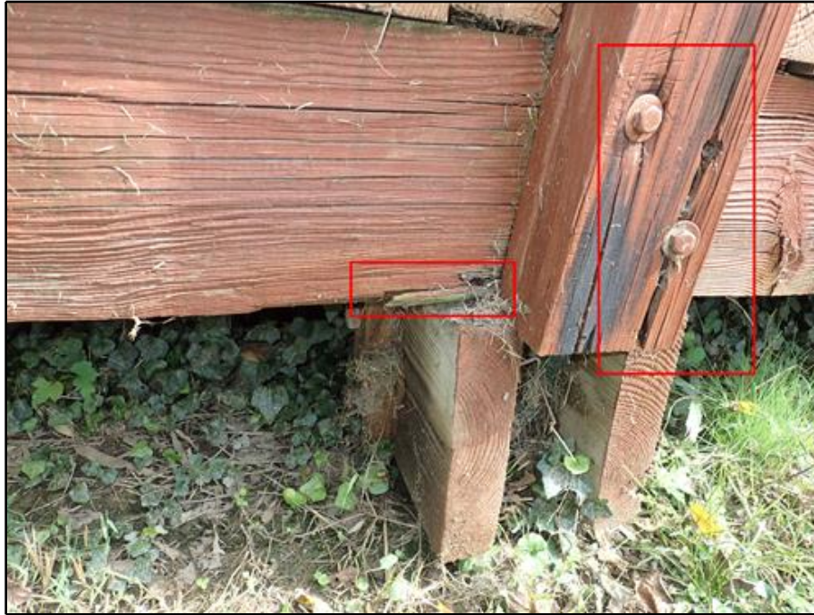
25. Typical Splintering at Fascia Stringer (Pier 12, South Side Shown) and Typical Open Checks at Hardware Connections
