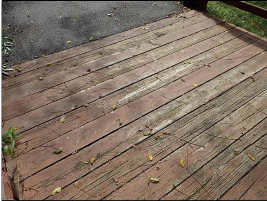
21. Span 14, Nine (9) Decayed Planks with Up to 1 in. Pick Penetrations
