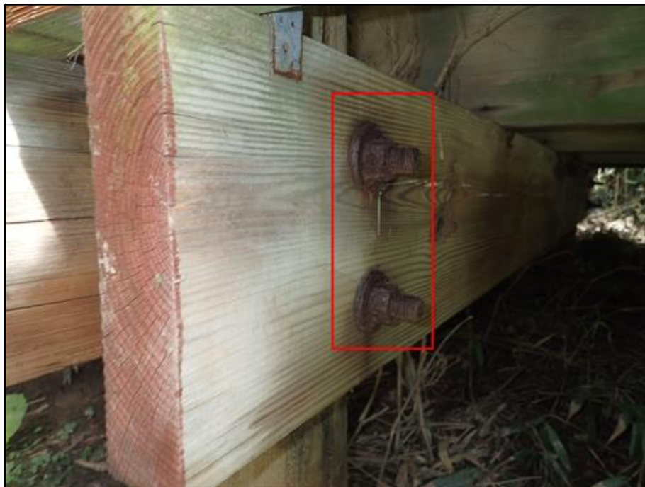
34. Typical Corrosion on Bent Cap Hardware
