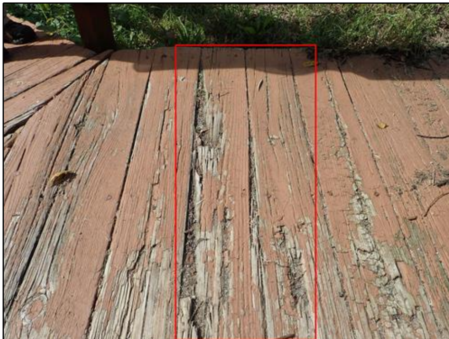
10. Span 1, Plank 7 - 6 ft. Long Area of Decay with Splintering and 1" Pick Penetrations
