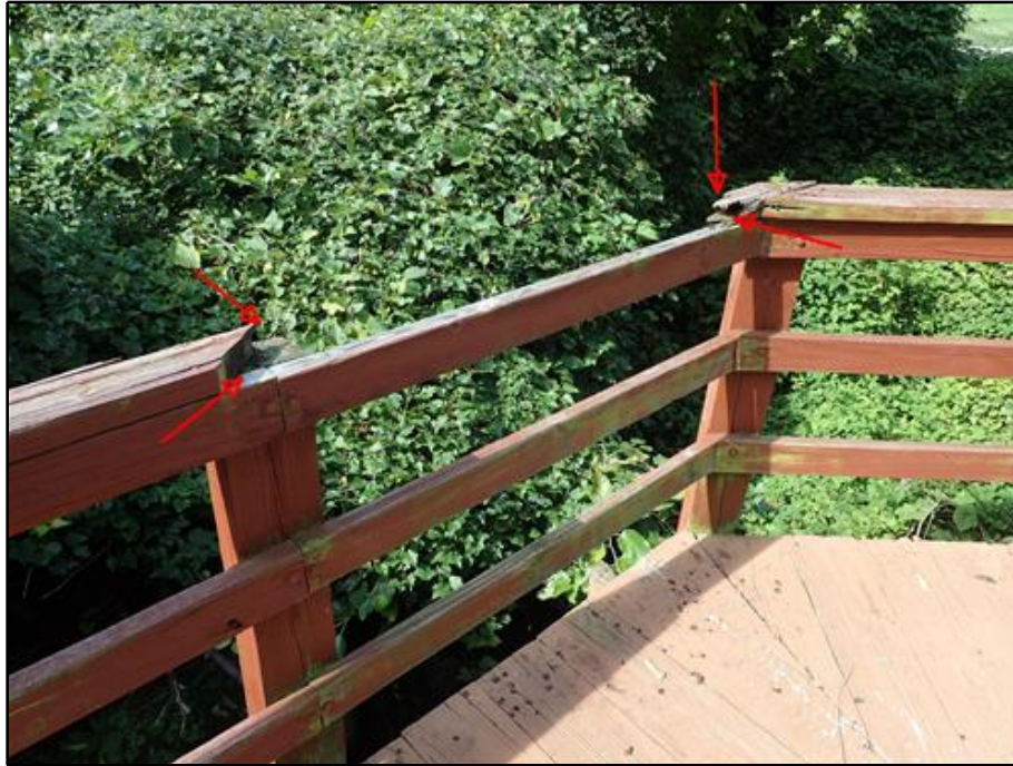
29. South Railing, Span 4 - 4 ft. Long Section of Top Cap Missing
