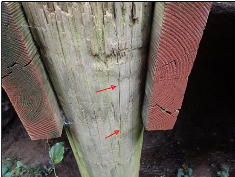
38. Typical 1/16 in. Open Checking in Pile (Bent 6 Shown)
