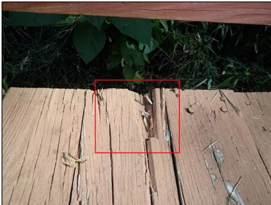
18. Span 12, Plank 5 - Exposed and Raised Nail with Adjacent Splintering
