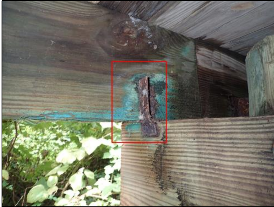
33. Heavy Corrosion on Stringer to Pile Cap Hardware
