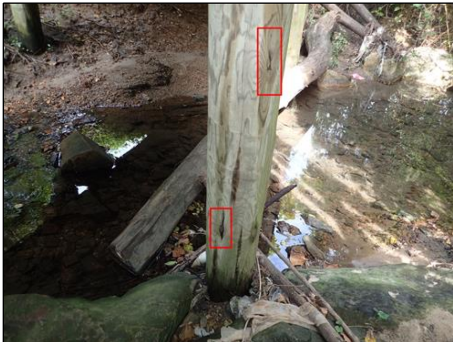
40. Bent 3, North Pile - Two (2) Areas of Decay with 1/2 in. Pick Penetrations up to 8 in. High
