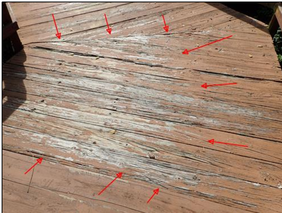
12. Heavier Wear on Deck Surface in Span 3
