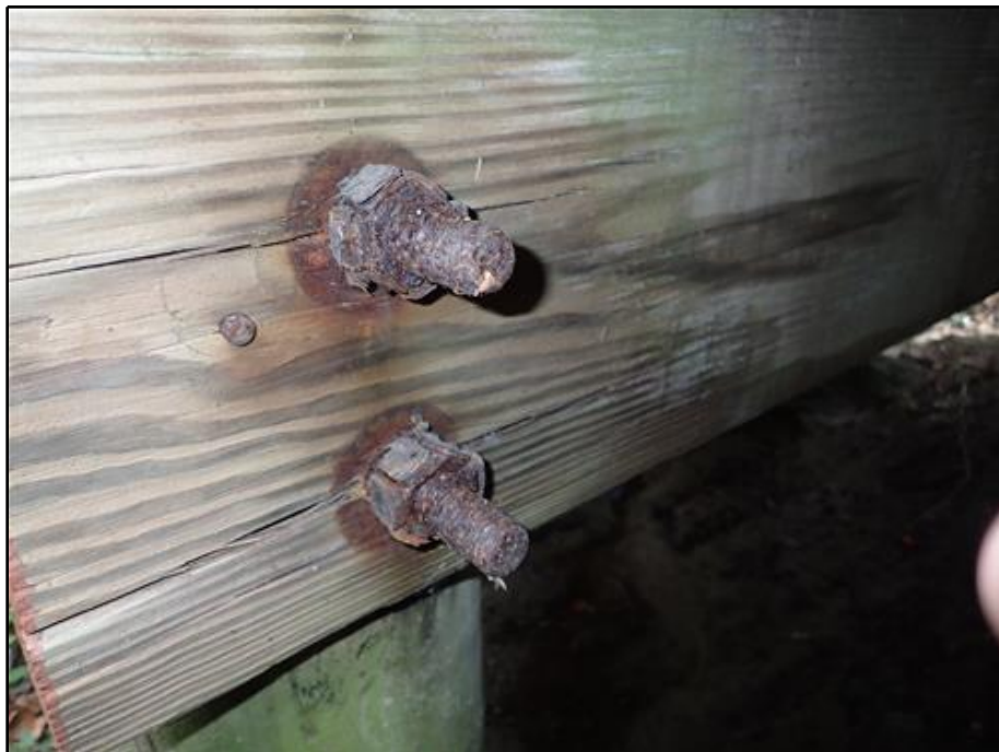
36. Heavier Corrosion on Pile Cap Hardware at Bent 5
