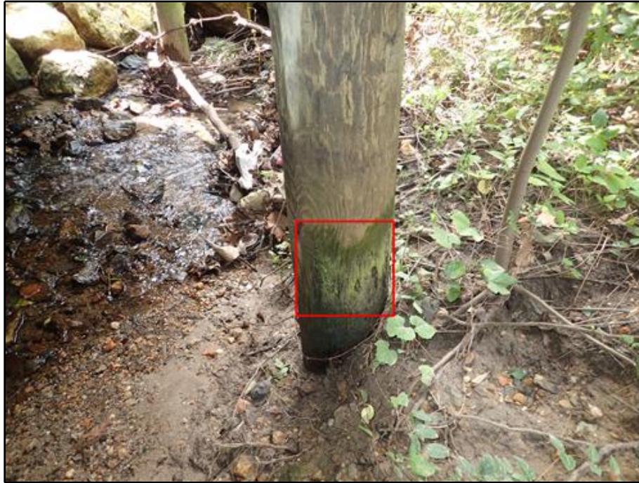
39. South Pile at Bent 2 - Up to 3/4 in. Pick Penetration at Base
