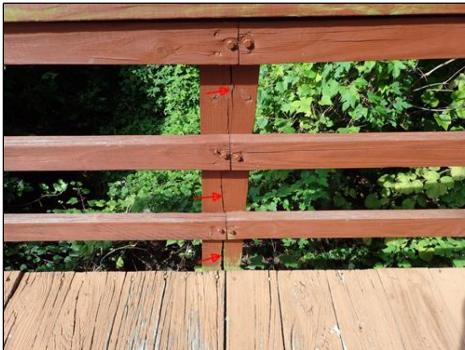
22. Typical Split at Post Connection - Span 3, Post 2
