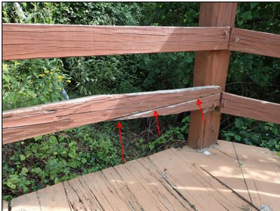
26. Span 1, North Railing - Splintered Section of Bottom Rail
