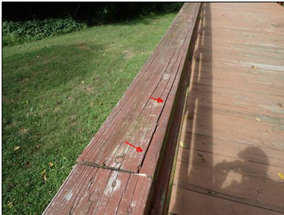
28. Typical, Up to 1/8 in. Open Checks in Top Cap of Railing
