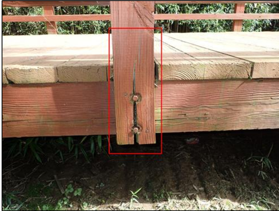
23. Typical Split in Railing (Span 9, Post 1, South Railing Shown)
