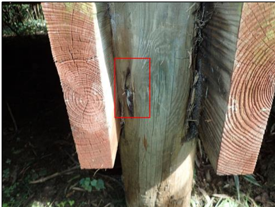
42. Bent 9, South Pile - Decay up to 1 ft. High x 3/4 in. Deep
