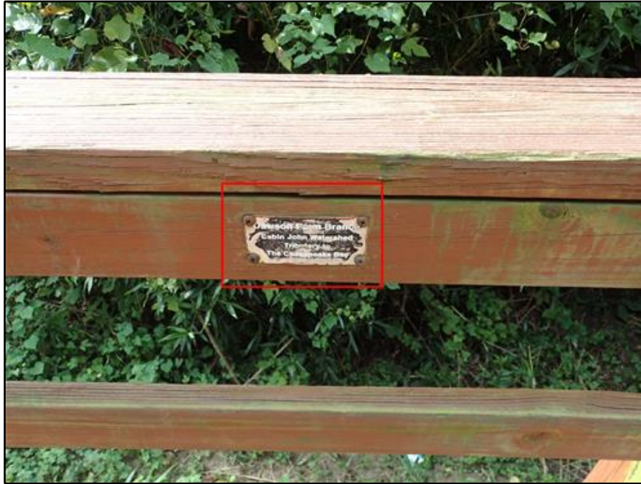
27. Worn Stream Name Plaque at South Railing
