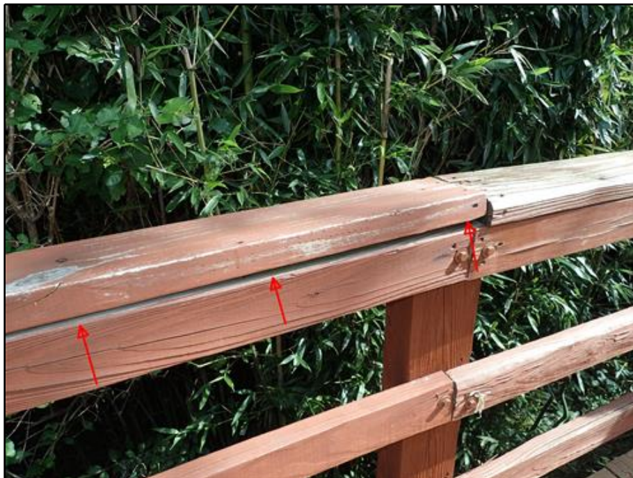
30. Span 7, North Railing - Top of Railing Cap Warped and Misaligned by 1 in.
