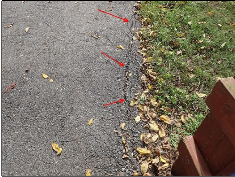
7. East Approach - 8 ft. Long x Up to 1/4 in. Open Crack in South Edge of Pavement
