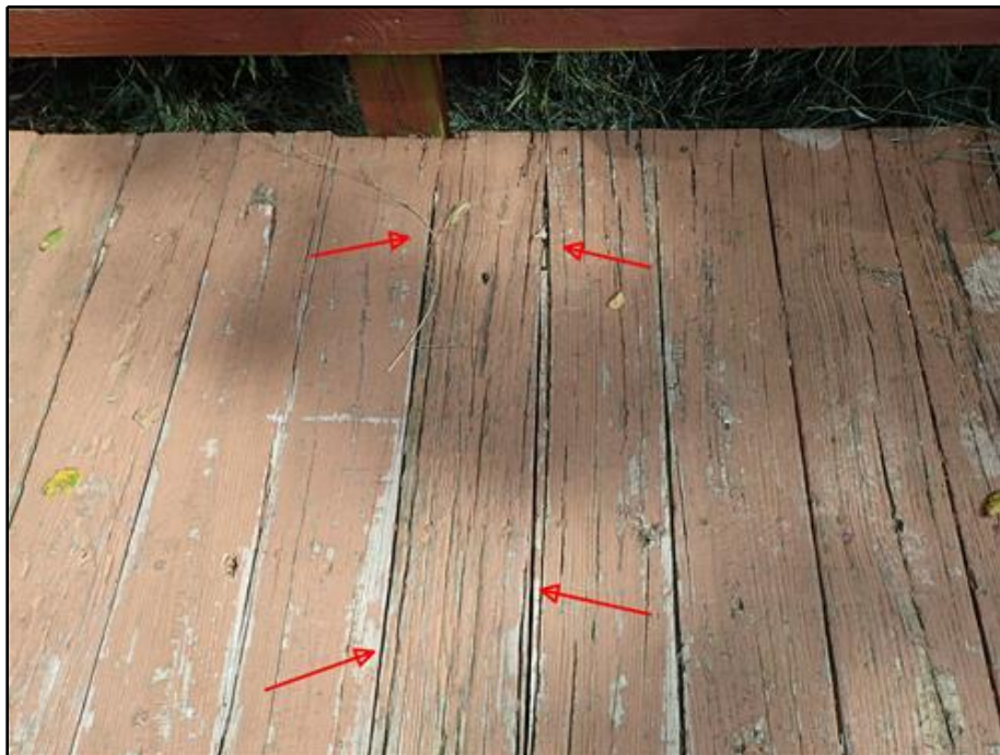
16. Span 11, Plank 1 - 4 ft. Wide Rot/Decay with 3/4" Pick Penetration
