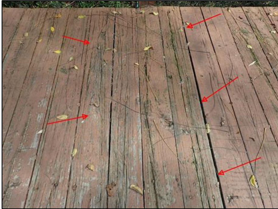
19. Spans 13 and 14, Decay in Planks with 1 in. Pick Penetration for a 3 ft. Width
