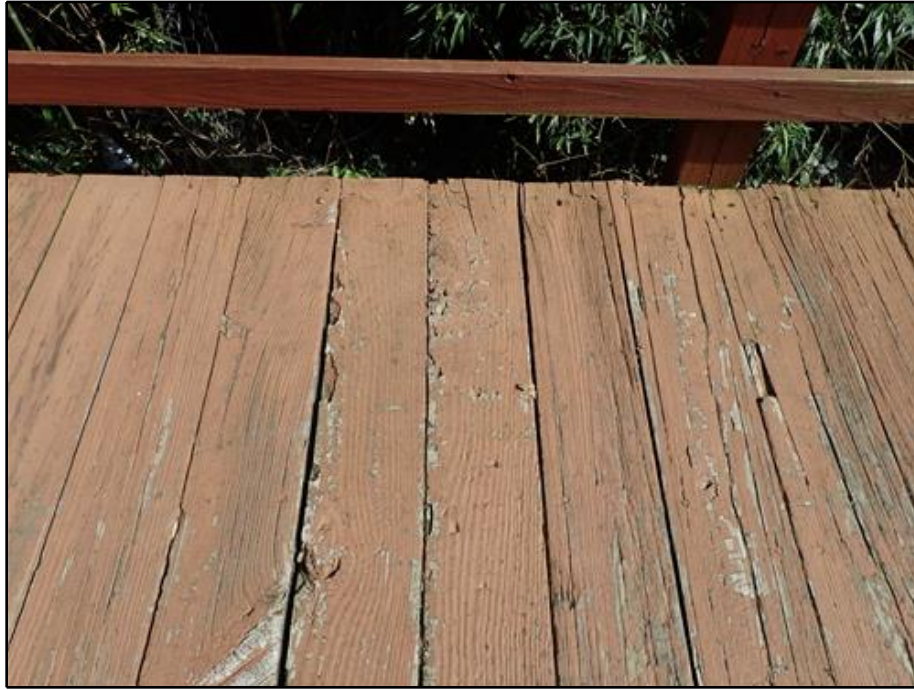
15. Span 10 - Decay in Planks 13 and 14 with 3/4" Pick Penetrations (Full Width)
