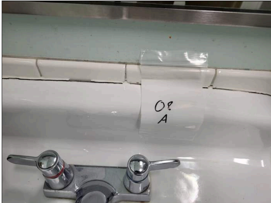
37 - White Bathroom Fixture Caulk
