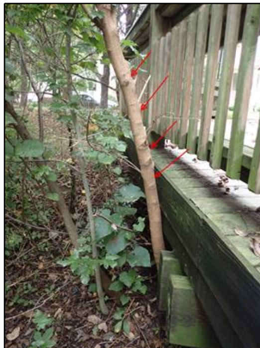
22. Approximately 4" Diameter Tree Growing under East Side of Span 15
