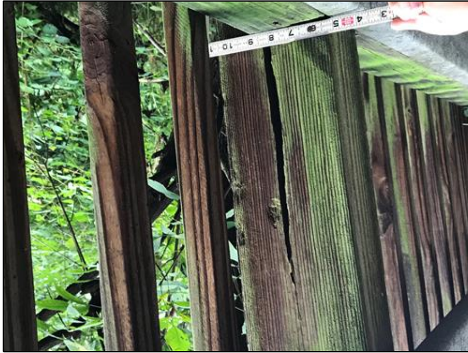
17. Up to 1 1/2" Open Split in 9th Wood Post from the South End of the East Railing
