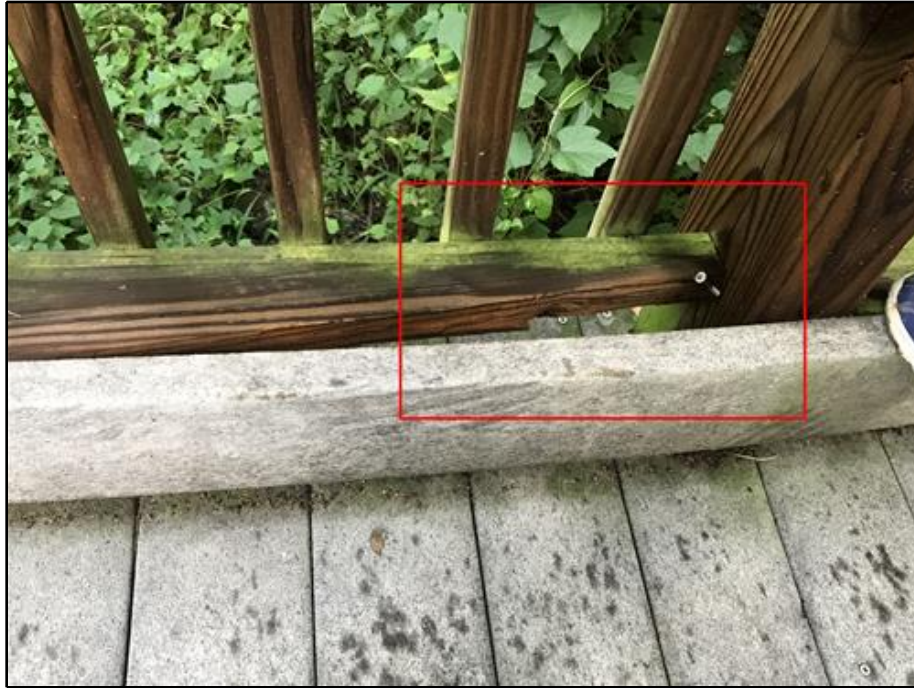
19. Broken Base Rail at 7th Post from North End of East Railing
