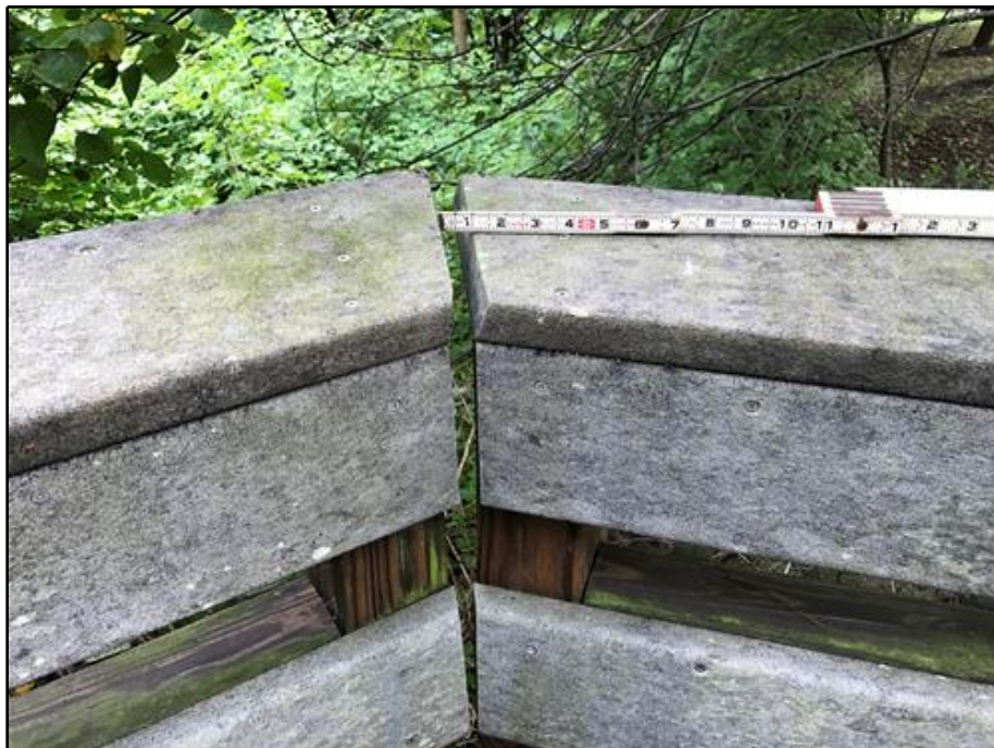
16. Typical Top Railing Gap Approximately 1" Separated
