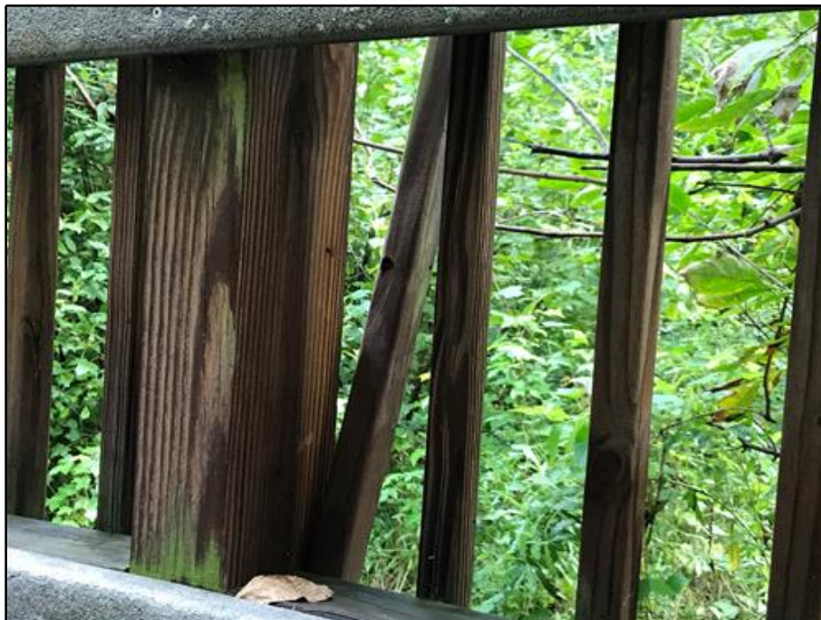
18. Loose Balustrade Adjacent to 10th Post from the South End of East Railing
