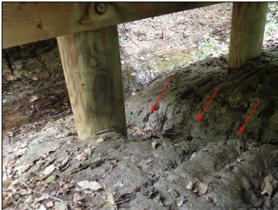
30. Erosion in Span 9 and 10 Leading to Channel Up to 10 Feet Long
