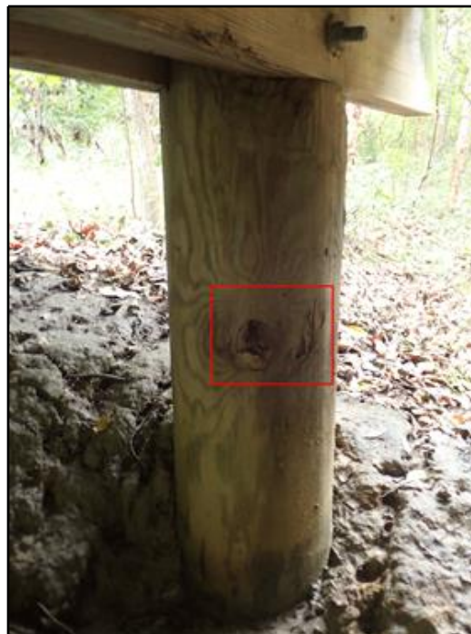
28. Approximately 3" High x 2" Wide x Up to 3/4" Pick Penetration Rot in west Pile at Bent 10
