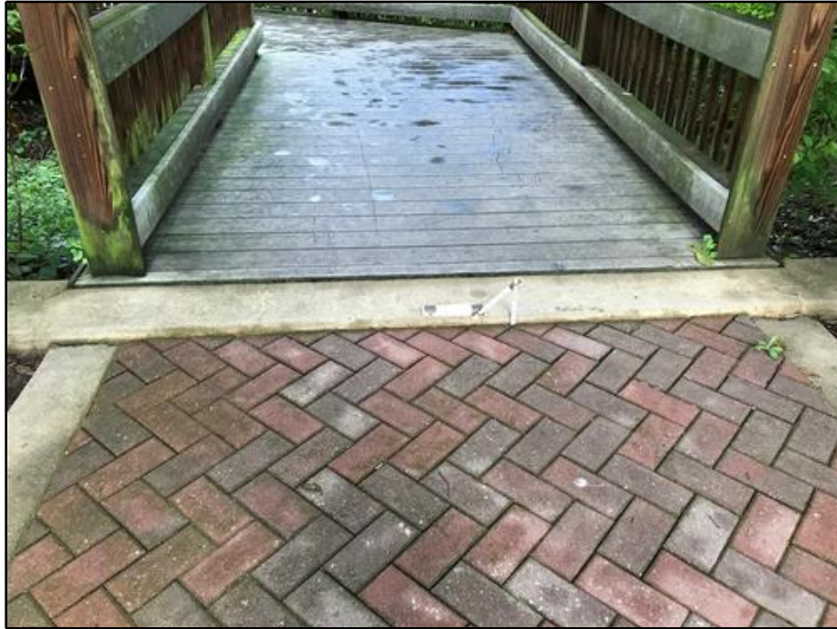
11. South Approach Walkway Transition Approximately 1 1/2" settled from Concrete Backwall
