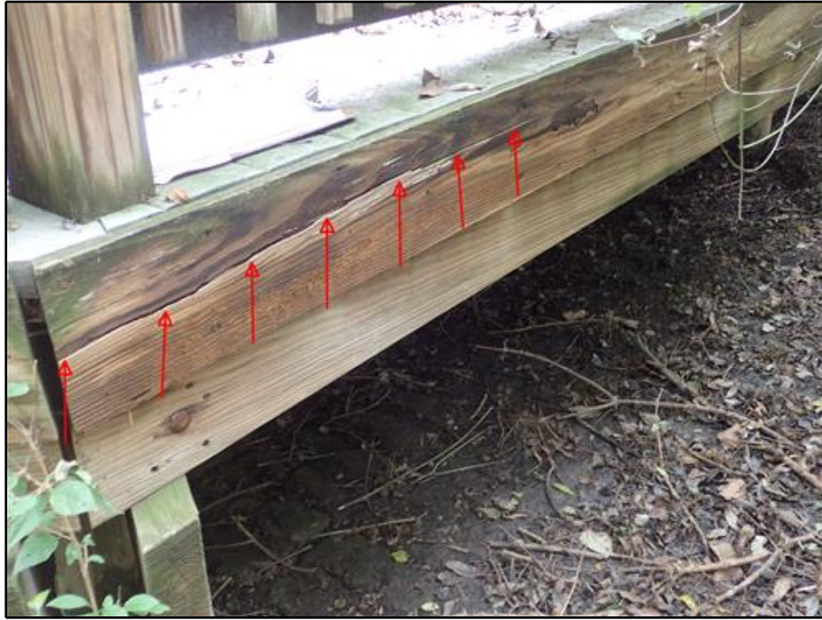
21. 3'-0" Long x 1/4" Open Splintering in Fascia Board at the West Side of Span 14
