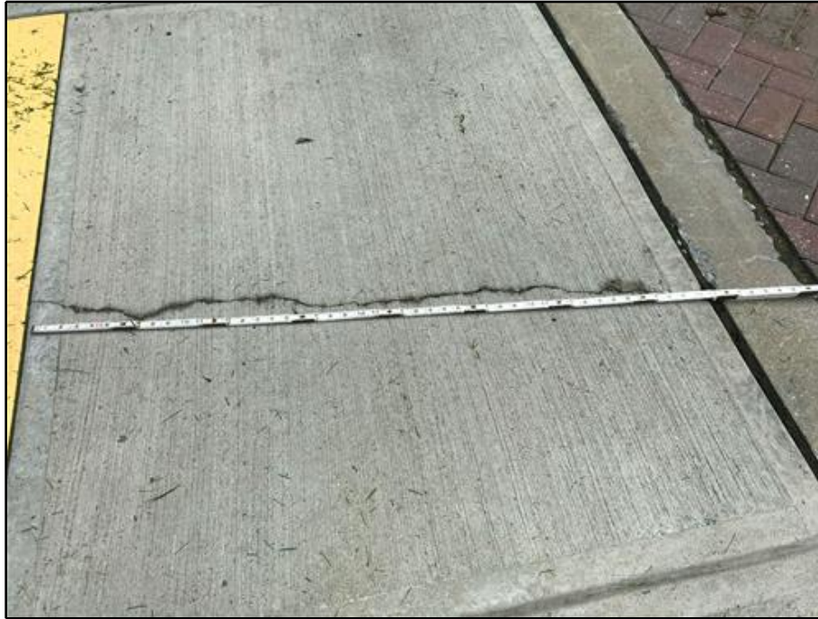
7. Approximately 3'-10" Long x 1/8" Open Crack in Concrete Sidewalk
