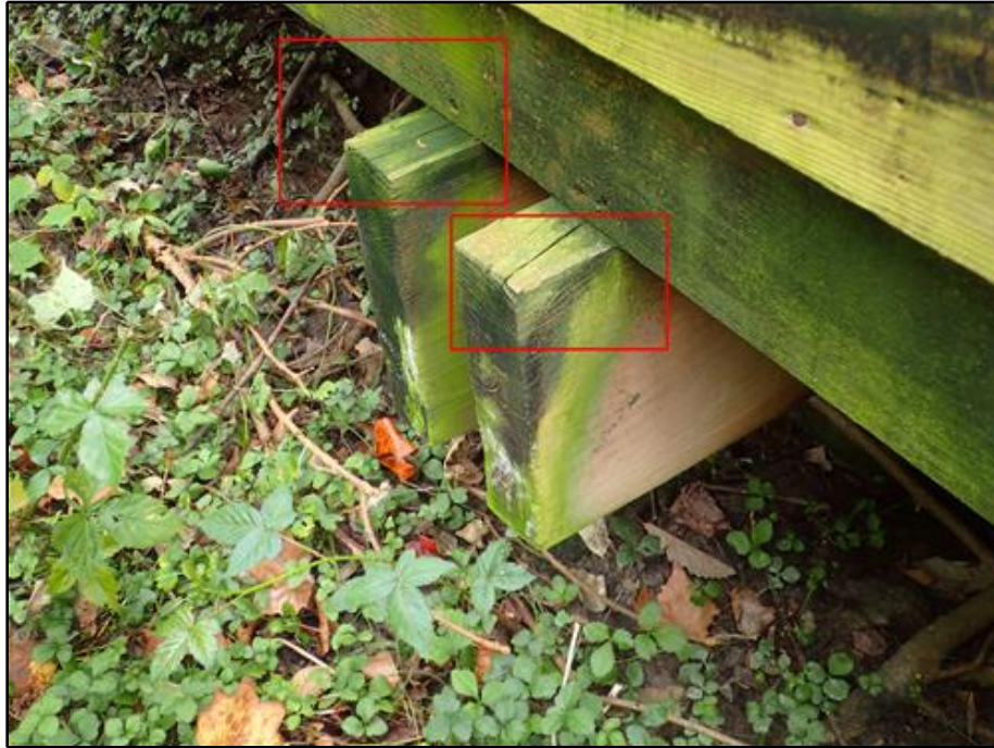
27. Typical Checks in Top of Timber Pile Caps (Bent 13 Shown)
