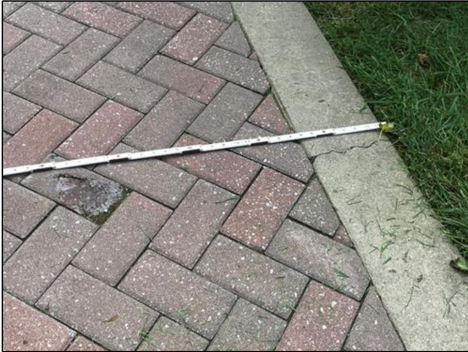
9. Hairline cracking in the North Approach at the West Side
