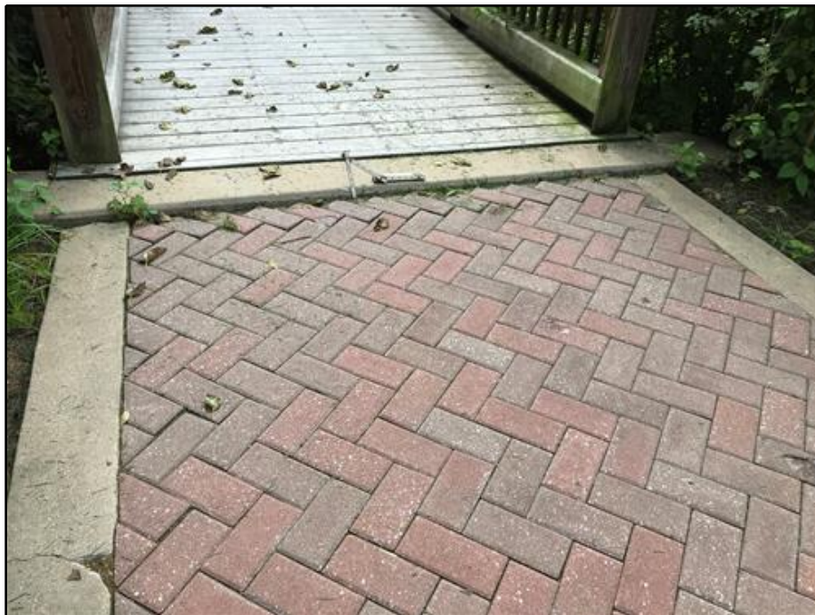
10. Up to 1 1/2" Settlement at the North Approach Concrete Backwall; Possible Trip Hazard
