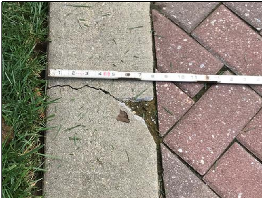
8. Hairline Cracking in the North Approach at the East Side
